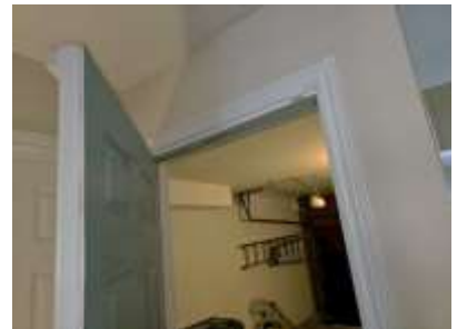
Pic. 27: Auto closer needed for garage entry door
