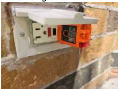
Pic. 7: Rear GFCI outlet defective
