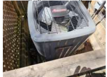
Pic. 6: AC unit 2008
