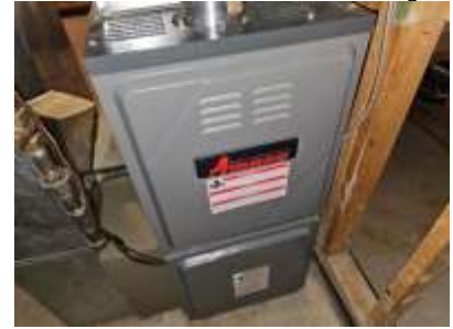
Pic. 33: Gas furnace 2008
