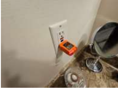
Pic. 19: GFCI outlet wired incorrectly
