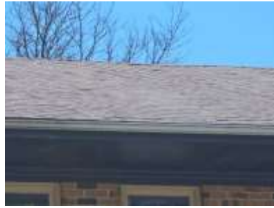
Pic. 2: Aging roof covering
