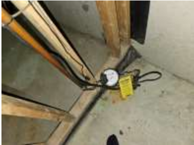
Pic. 34: Water main
