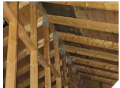
Pic. 12: Some sheathing noticeable discoloured
