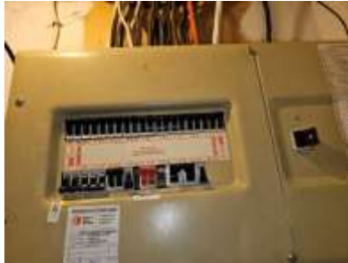
Pic. 35: 200 amp breaker panel
