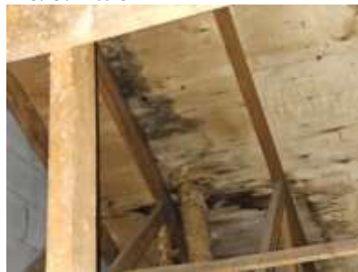
Pic. 11: Old water stains and apparent visible mould growth
