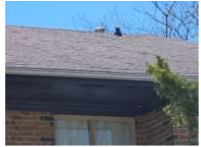
Pic. 3: Aging roof covering
