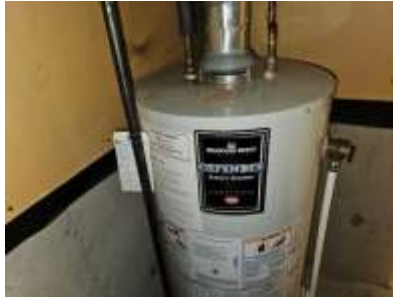
Pic. 32: Rental hot water tank 2008
