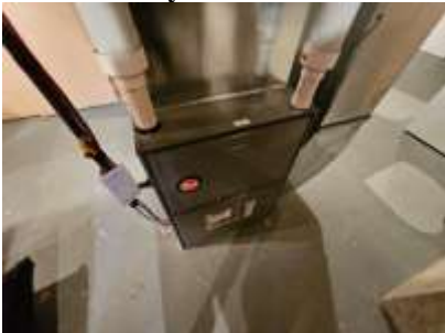
Pic. 37: Gas furnace 2013
