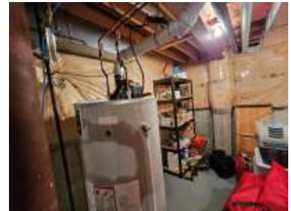
Pic. 36: Hot water tank 2019
