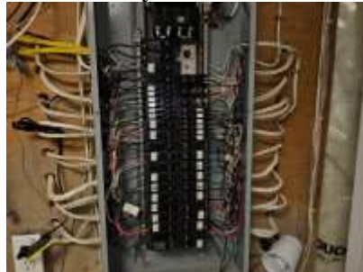
Pic. 38: 200 amp breaker panel
