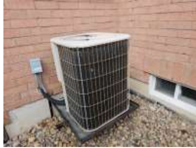
Pic. 5: AC unit 2000
