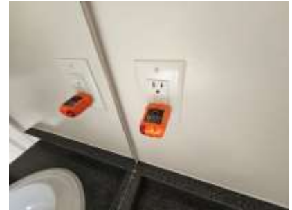
Pic. 21: GFCI outlet won't trip – replace
