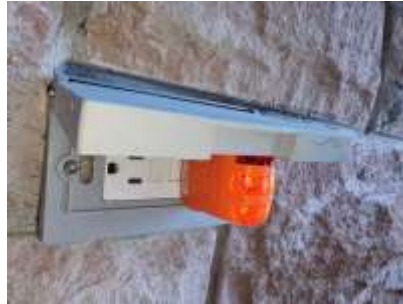
Pic. 8: Front GFCI won't trip – replace
