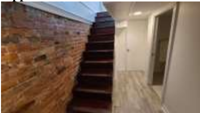
Pic. 28: Recommend adding a handrailing for basement stairwell
