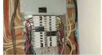
Pic. 24: 125 amp breaker panel
