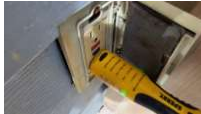
Pic. 8: Rear GFCI outlet wont trip and should be replaced
