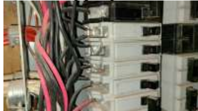
Pic. 26: Several breakers double tapped
