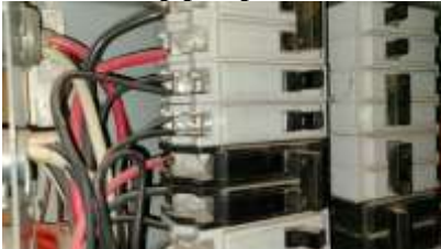
Pic. 25: Several breakers double tapped
