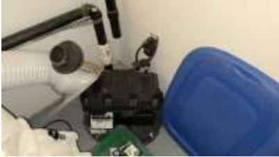
Pic. 22: Sump pump #1
