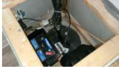
Pic. 23: Sump pump #2
