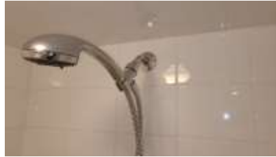
Pic. 20: Water leak at handle pipe connection
