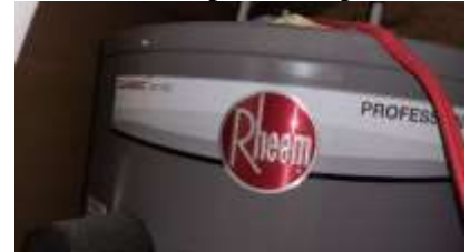
Pic. 27: Electric hot water tank 2017
