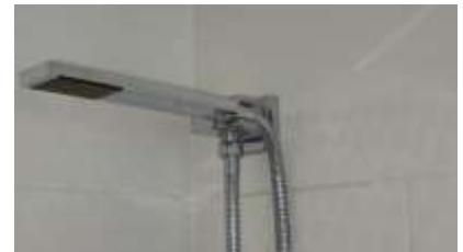
Pic. 12: Water leak at handle pipe connection
