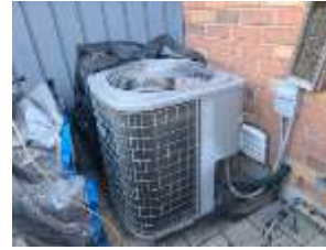
Pic. 3: AC unit 2006
