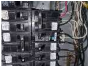
Pic. 34: Bedroom ARCF breaker defective and needs to be replaced
