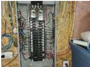
Pic. 33: 200 amp breaker panel
