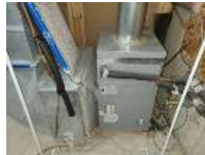
Pic. 31: Hot water furnace
