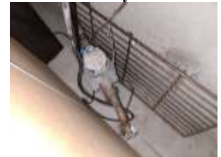
Pic. 32: Water main
