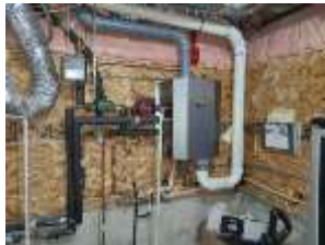
Pic. 30: Tankless hot water boiler
