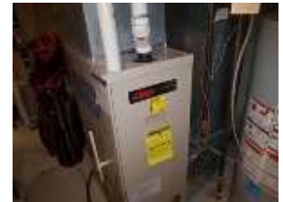
Pic. 32: High efficiency gas furnace 2002
