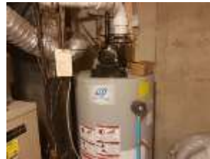
Pic. 31: Newer hot water tank
