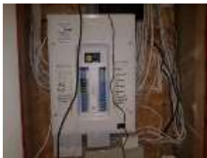
Pic. 33: 100 Amp breaker panel with all copper wire
