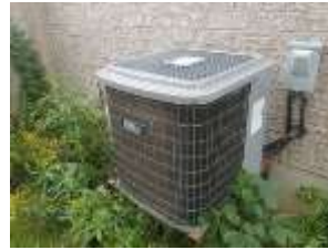
Pic. 3: AC unit 2002
