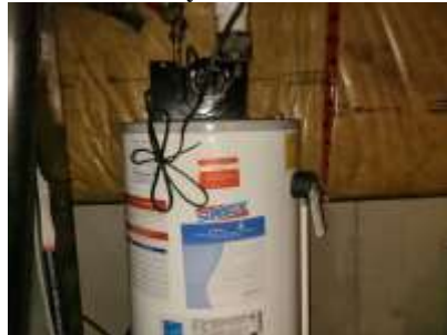
Pic. 26: Rental hot water tank
