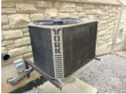
Pic. 4: AC unit 2007
