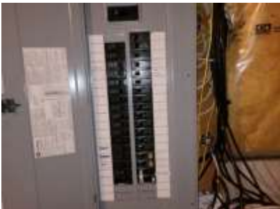
Pic. 28: 200 amp breaker panel with all copper wire
