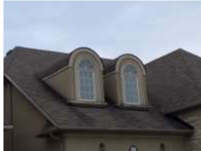
Pic. 2: Roof covering aging
