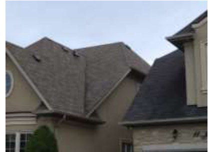
Pic. 3: Roof covering aging
