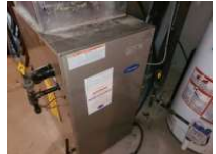
Pic. 27: Gas furnace 2006
