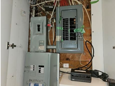
Pic. 34: 100 amp breaker panel and pony panel
