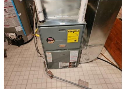
Pic. 33: Gas furnace 2008
