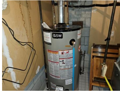
Pic. 32: Rental hot water tank 2018
