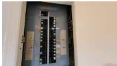
Pic. 32: 100 amp breaker panel
