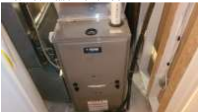
Pic. 31: Gas furnace 2014
