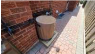
Pic. 4: AC unit – old – cover could not be reviewed
