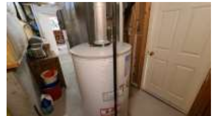
Pic. 30: Rental hot water tank 2008
