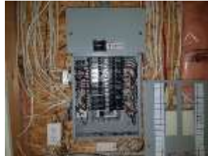
Pic. 26: 100 amp breaker panel with all copper wire
