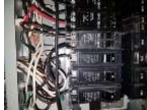
Pic. 27: 20 amp breaker appears oversized for the wire size
