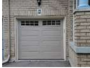
Pic. 3: Garage – No access
