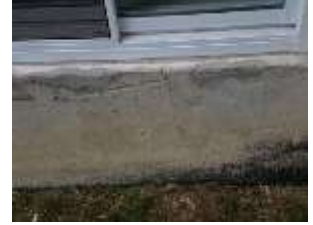
Pic. 4: Typical foundation crack
