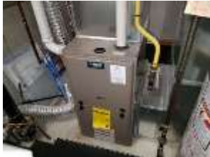
Pic. 25: Updated high efficiency gas furnace
