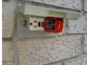
Pic. 7: Rear GFCI outlet needs replacement
