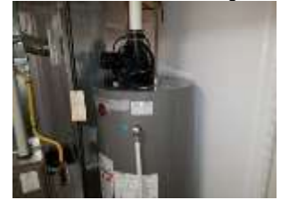
Pic. 24: Rental hot water tank
