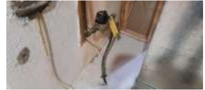
Pic. 27: Water main
