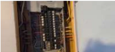
Pic. 28: 100 amp breaker panel
