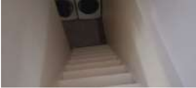
Pic. 22: No hand railing in basement stairwell
