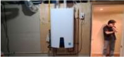
Pic. 25: Tankless hot water system 2016
