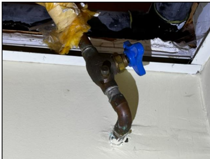
25. Hosebib shut off valve
