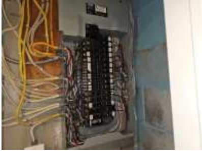
Pic. 31: 100 amp breaker
