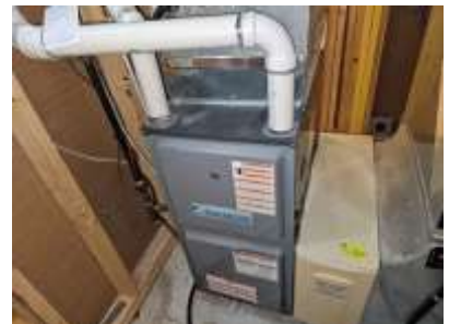
Pic. 30: Gas furnace 2021
