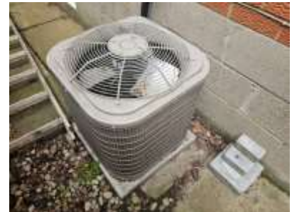
Pic. 9: AC unit 2014
