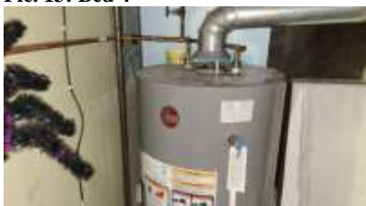
Pic. 16: Hot water tank 2015
