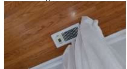
Pic. 30: Asbestos based wrapping present around the floor register heat boots
