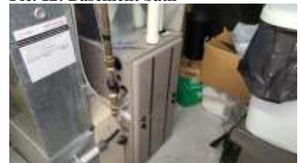
Pic. 15: Gas furnace 2009
