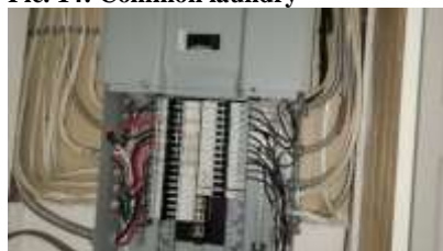
Pic. 17: 200 amp breaker panel
