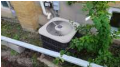
Pic. 7: AC unit 1998
