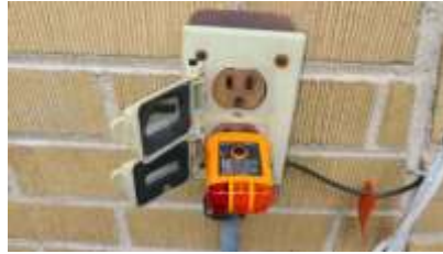
Pic. 2: Exterior outlet wired incorrectly
