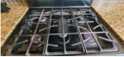
Pic. 25: Gas stove middle burner would not ignite
