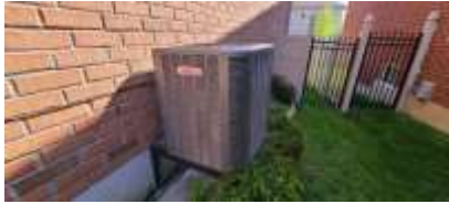
Pic. 4: AC unit 2022
