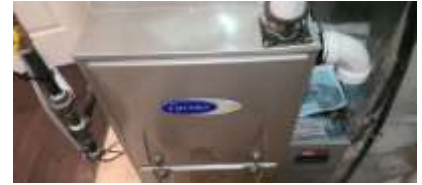
Pic. 36: Gas furnace 2019
