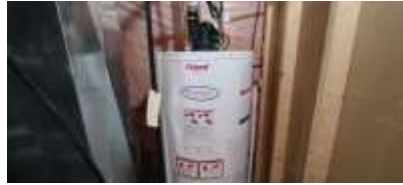
Pic. 35: Rental hot water tank 2022
