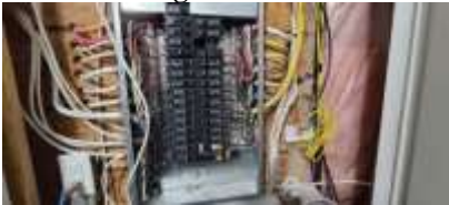
Pic. 37: 100 amp breaker panel
