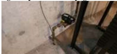
Pic. 32: Water main
