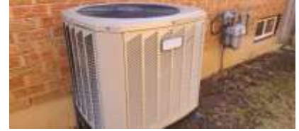
Pic. 3: AC unit 2012
