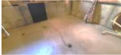
Pic. 29: Foundation repair and signs of past water seepage issue
