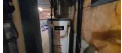
Pic. 30: Rental hot water tank 2006
