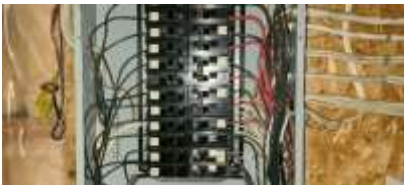
Pic. 34: All copper wire
