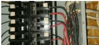
Pic. 35: Dryer breaker oversized should be a 30 amp breaker (old practice)
