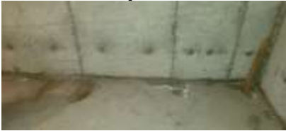
Pic. 28: Signs of past moisture issues
