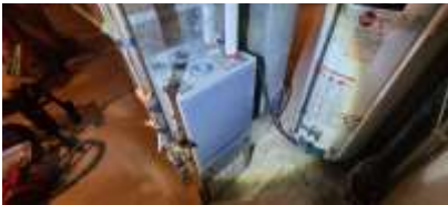
Pic. 31: Gas furnace 2009
