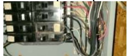
Pic. 36: Double tapped breaker
