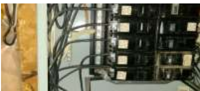
Pic. 37: Double tapped breaker
