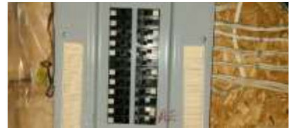
Pic. 33: 100 amp breaker panel
