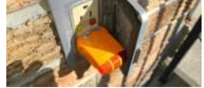
Pic. 6: Rear GFCI outlet wired incorrectly
