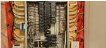
Pic. 31: 100-amp breaker panel
