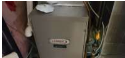
Pic. 29: Gas furnace 2010
