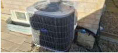
Pic. 4: AC unit 2009
