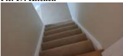
Pic. 22: Handrailing needed for basement stairwell
