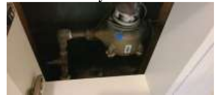
Pic. 30: Water main
