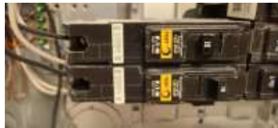
Pic. 32: Both ARCF breakers need to be replaced
