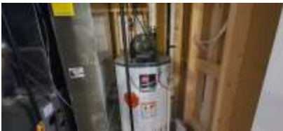
Pic. 28: Hot water tank 2009
