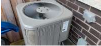
Pic. 4: AC unit 2017
