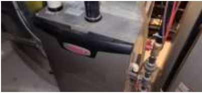
Pic. 25: Gas furnace 2017
