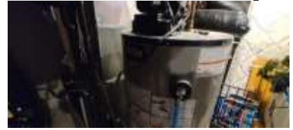
Pic. 24: Rental hot water tank 2017
