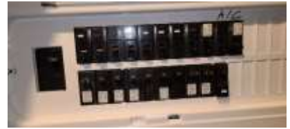
Pic. 27: 100 amp breaker panel
