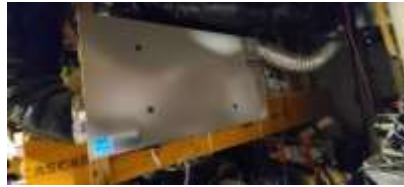
Pic. 26: HRV system
