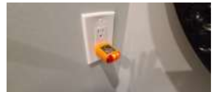
Pic. 21: Outlet in bathroom need to be GFCI protected
