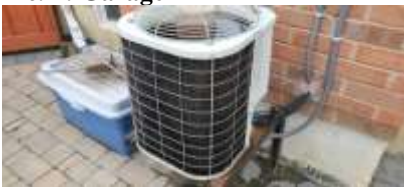
Pic. 7: Original AC unit
