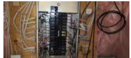
Pic. 33: 100-amp breaker panel
