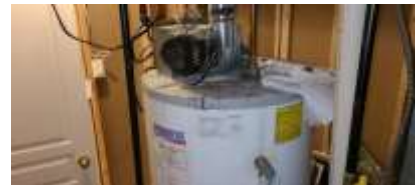
Pic. 30: Retnal hot water tank
