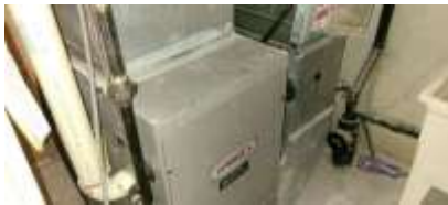
Pic. 31: Original gas furnace
