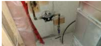
Pic. 32: Water main
